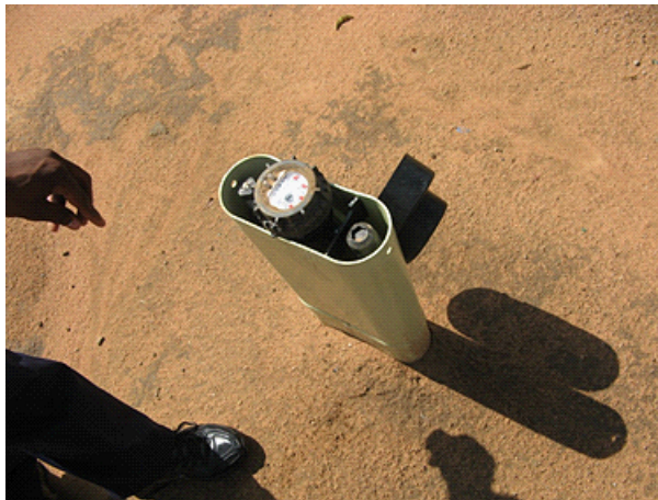
FIGURE S1.—Water meter.
